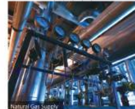
Natural Gas Supply
